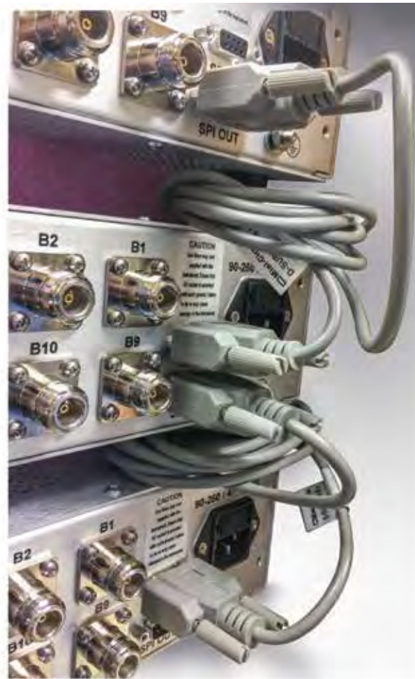
3 ZTDAT racks “daisy chained” via SPI ports
