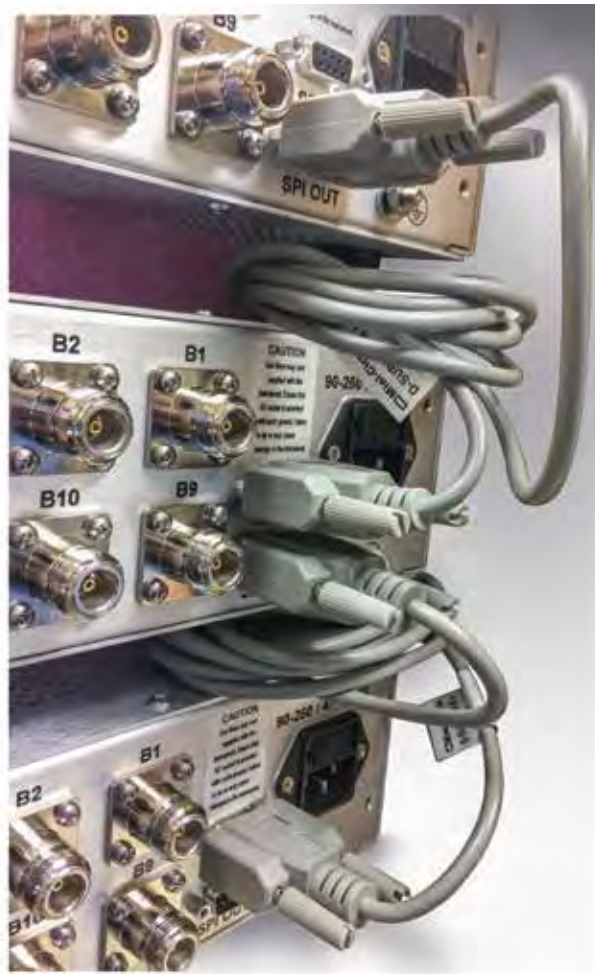
3 ZTDAT racks “daisy chained” via SPI ports
